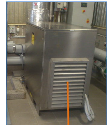
Biogas Compressor (not supplied by Ansaldo)
