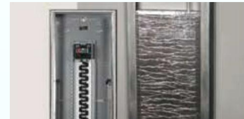
Electrical Panel Box
