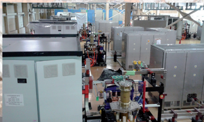
Nidec ASI scope of supply during commissioning
