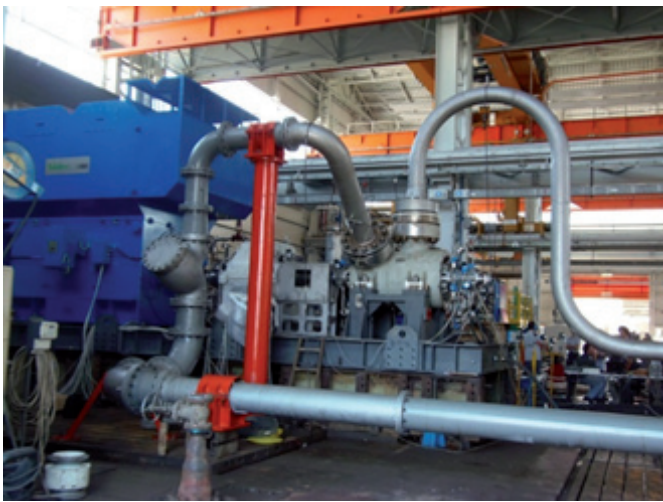
Fig. 8– Main Injection Pump (MIP), CT 900 Y4 induction motor, gearbox, suction & discharge tubing during string test at Termomeccanica Pompe
