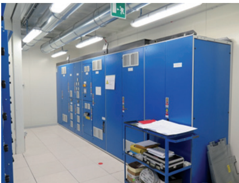
Fig. 5 - Variable frequency converter, type SVTN, mounted inside the Local Equipment Room (LER)
