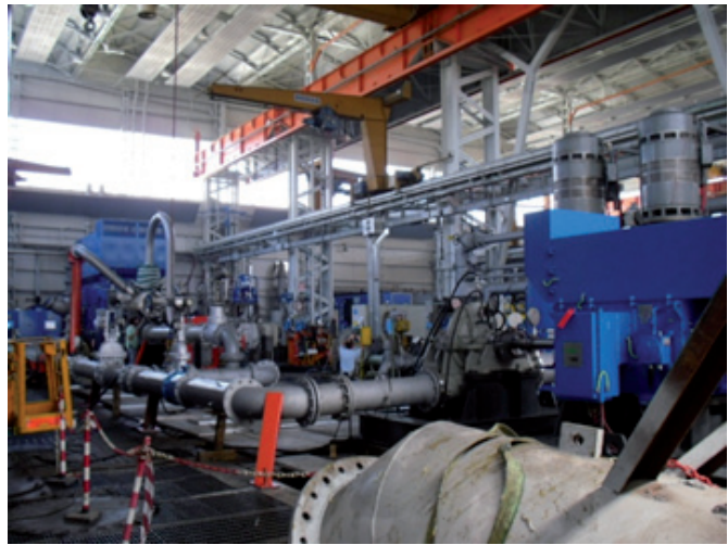
Fig. 9 – Booster Pump (BP) and CT 400 Y4 induction motor (front right) connected to main injection pump and CT 900 Y4 induction motor (back left) during string test at Termomeccanica Pompe
