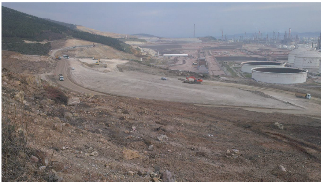
Fig. 3 - South view with new naphtha tanks
