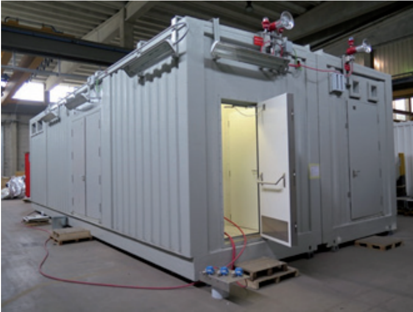
Fig. 6– The Local Equipment Room (LER) during assembly
