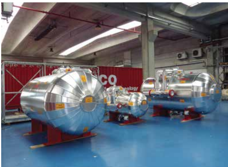
Fig. 5 - Uzbekistan project: foam bladder tanks with thermal insulation for very low temperature
