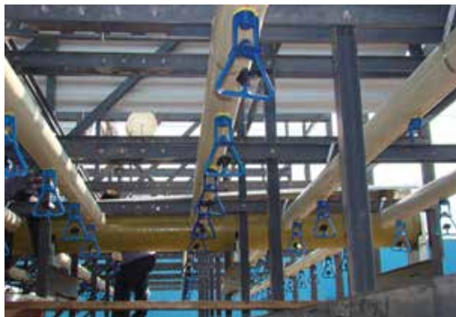
Fig. 4 - Ecojet® nozzles installed inside a cooling tower
