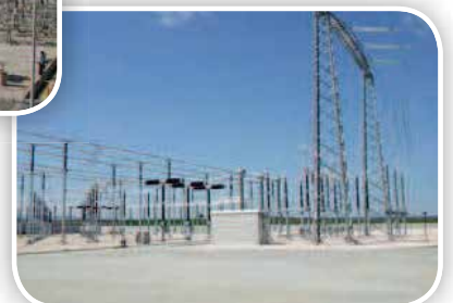
400kV AIS Italy
