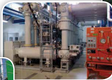
150kV GIS Belgium
