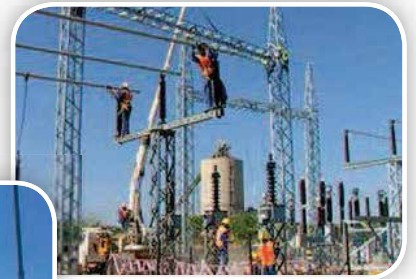
110kV AIS Mozambique
