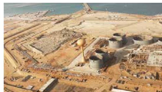
General view of the Jeddah South Thermal Power Plant, in Saudi Arabia
