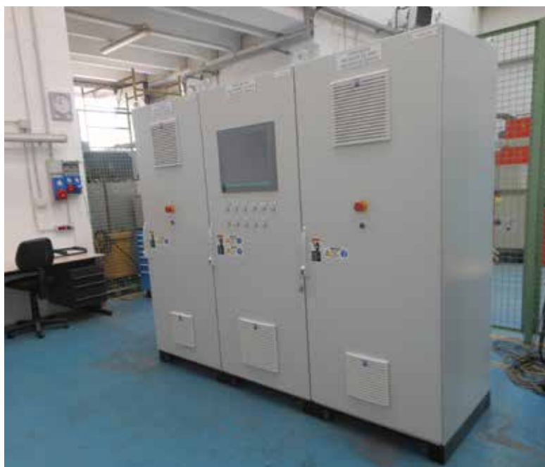
Fig. 2 – The PLC control panel for the job in Mexico
