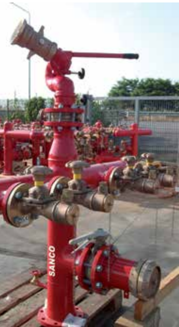
Fig. 3 – Kuwait project: fire monitor on hydrant
