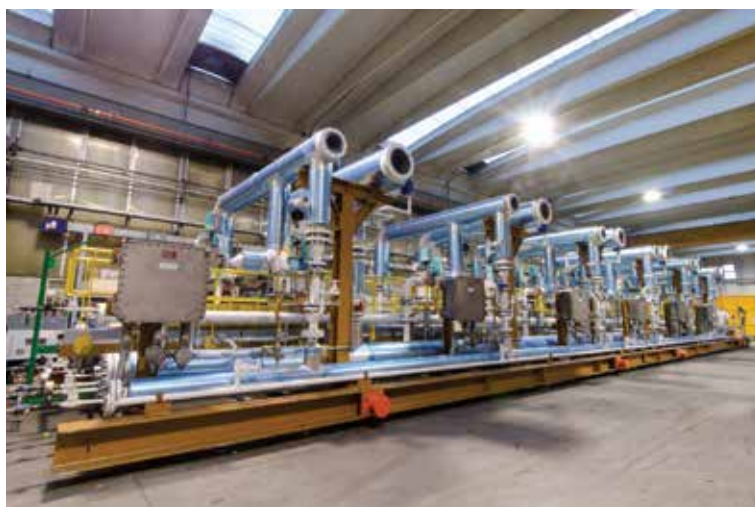
Fig. 1 - Skid PSA unit
