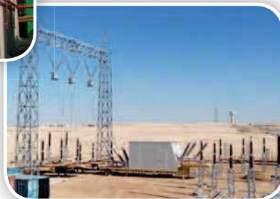
400/220kV Mobile Algeria
