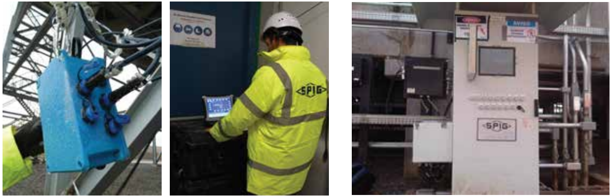
Fig. 11 - Unico installed on an ACC and a CT for predictive maintenance
