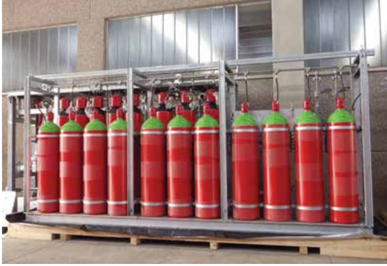
Fig. 2 – Kuwait project: gaseous systems
