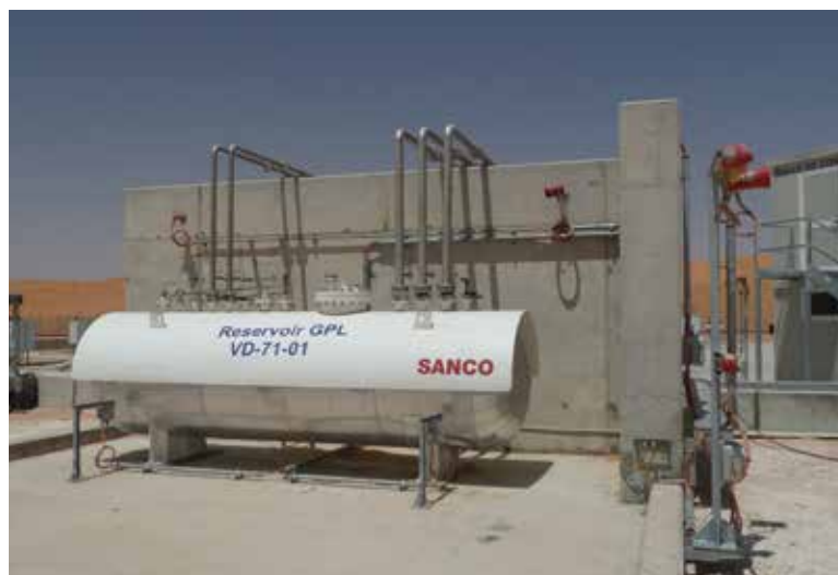
Fig. 7 - Fire training ground LPG vessel
