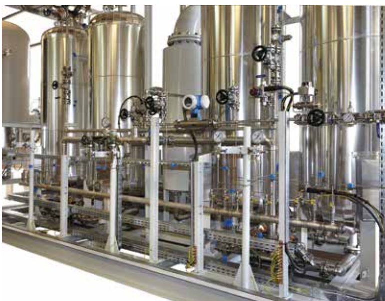
Fig. 3 - Close-up of PSA oxygen generation plant
