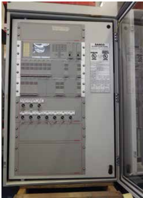
Fig. 4 – Kuwait project: fire & gas detection panels (UL listed)
