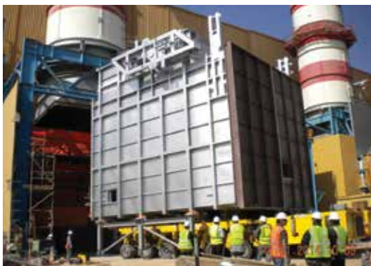
Fig. 1 - Ras Abu Fontas A2 (Qatar): diverter and guillotine dampers fully preassembled and tested in Dubai
