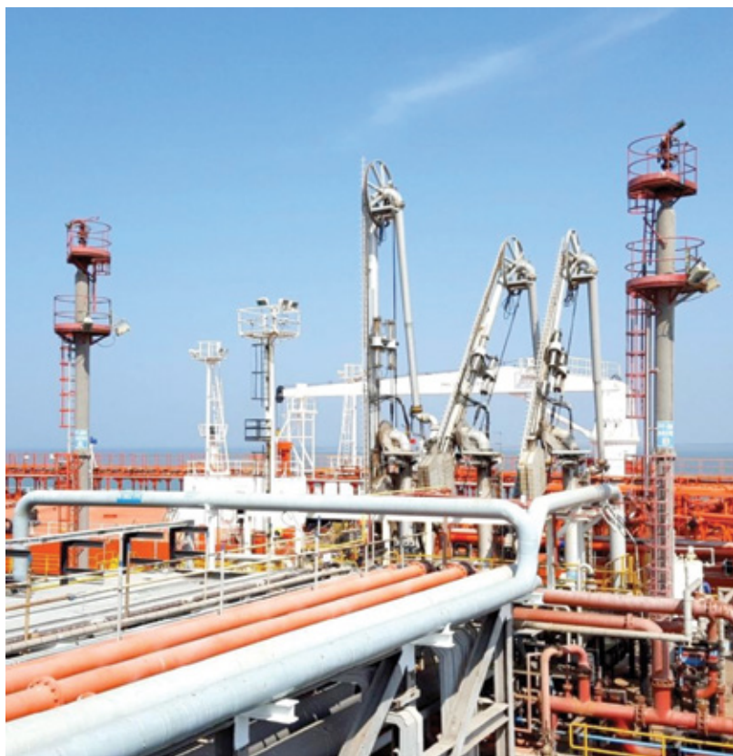
Remote controlled monitors on towers
