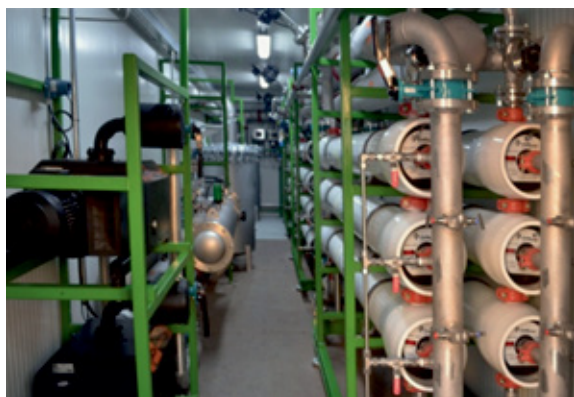
Figure 1. Membrane Deaeration skid
