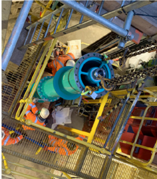
(left) New pump descending into the shaft (right) new pump being lifted into place Courtesy of Stantec - IMAGE
