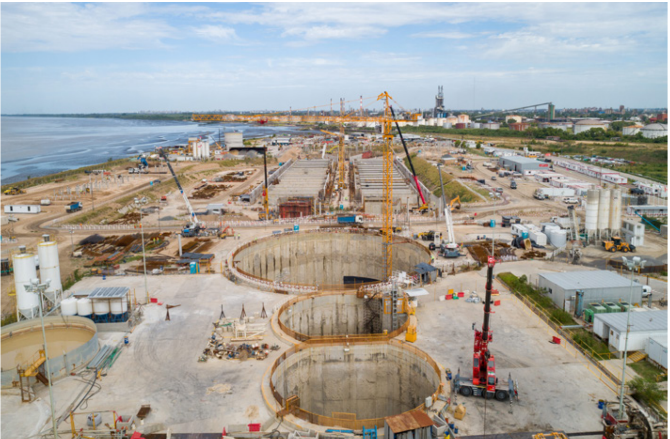
Lot of the Riachuelo System in Buenos Aires, Argentina (Fisia Italimpianti)
