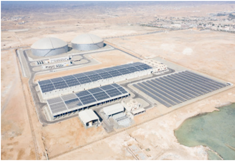
Figure 5: PV installation in SWRO plant
