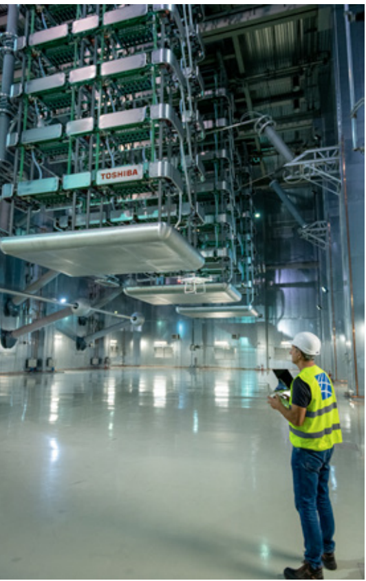
Italy-Montenegro HVDC link - Kotor converter station valve hall
