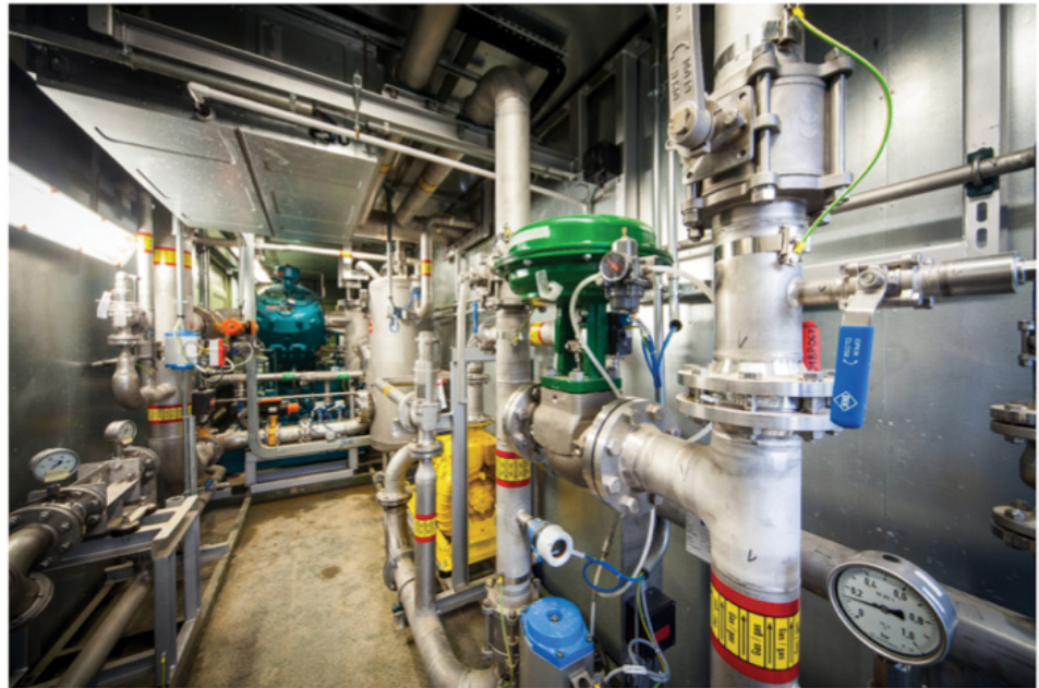
Figure 14: South Milford AD plant (UK) – Compressor
