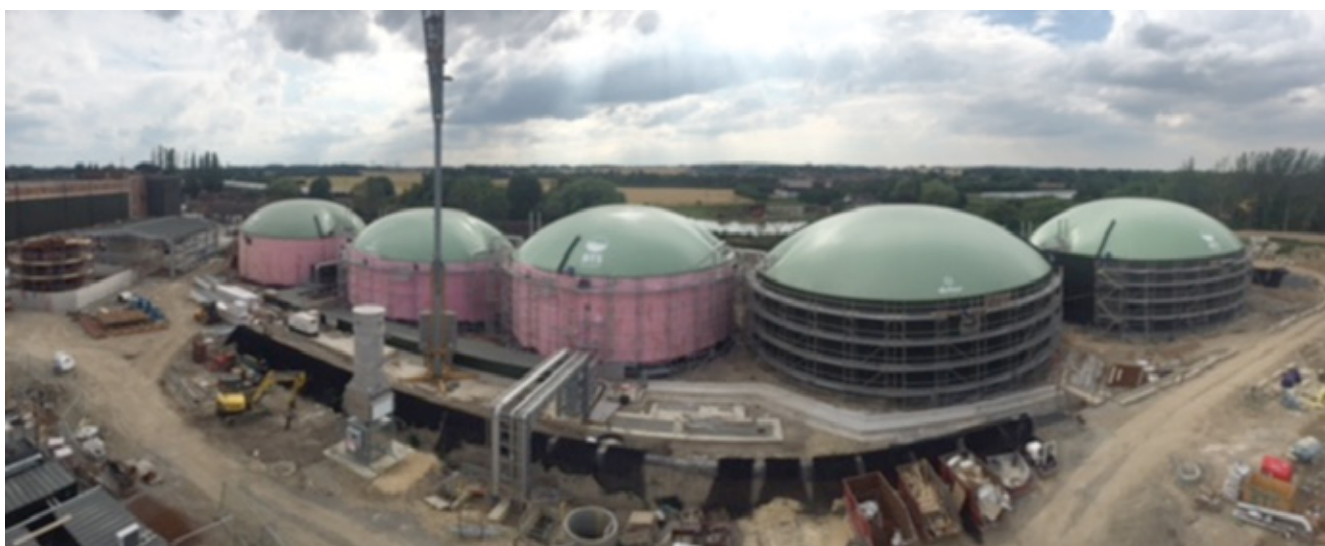
Figure 4 - South Milford AD plant (UK) – After 9 months from the start of the Project
