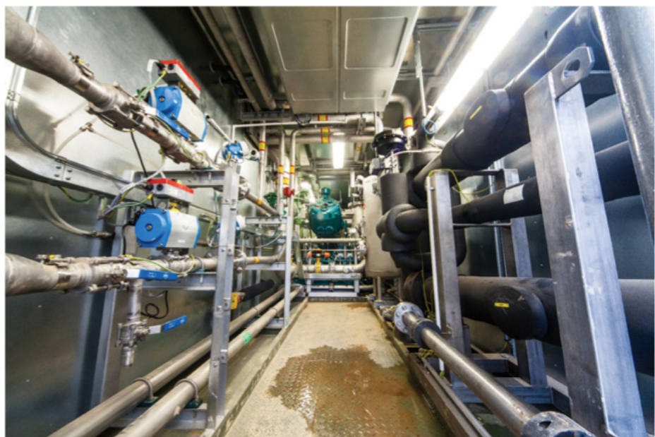
Figure 15: South Milford AD plant (UK) – Compressor 2
