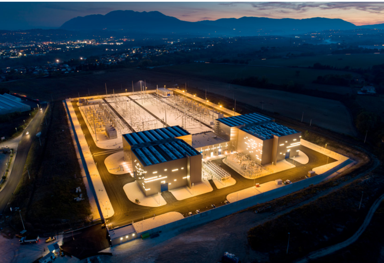
Italy-Montenegro HVDC link - Cepagatti converter station
