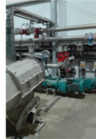
Pipework and Pumping
