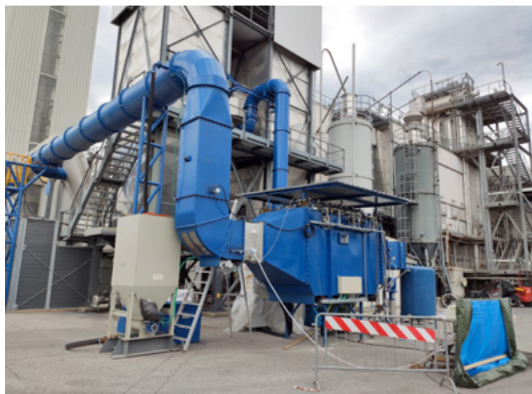
Figure 4 - WES installation in a Waste to Energy (WTE) plant
