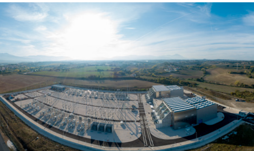
Italy-Montenegro HVDC link - Cepagatti converter station
