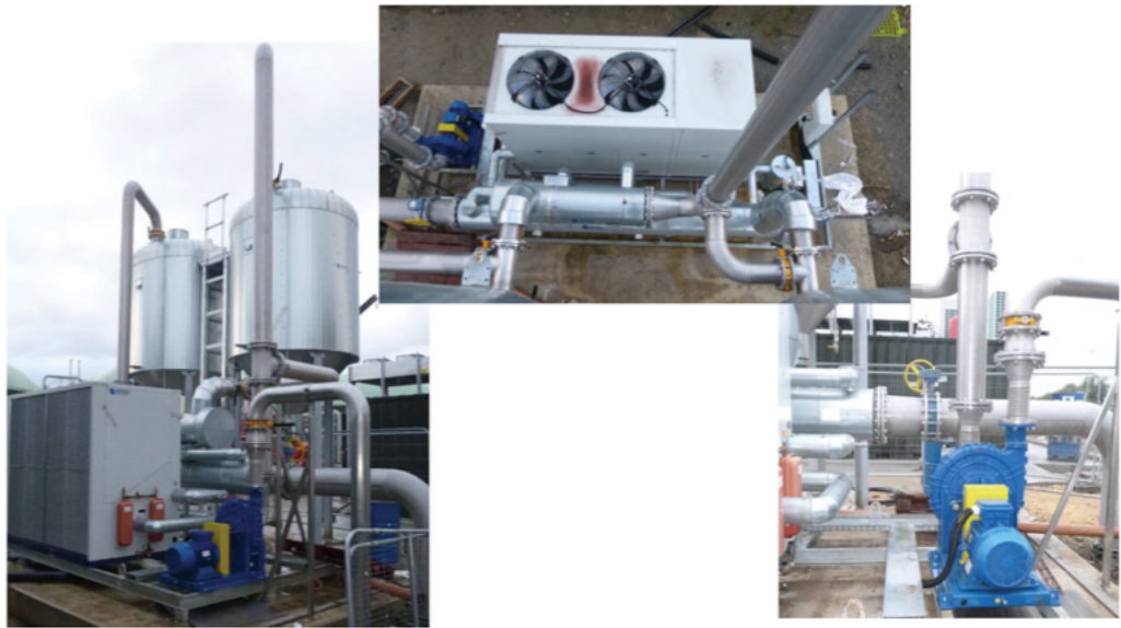
Figure 10 - South Milford AD plant (UK) – Equipment for emission reduction
