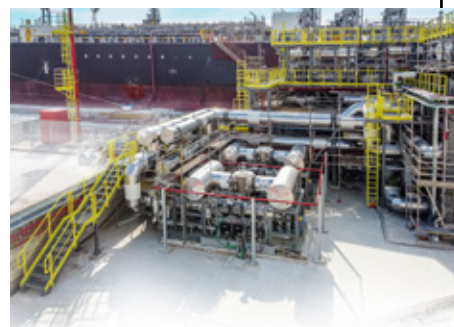
Courtesy of Depositi Italiani GNL DIG, Ravenna, Italy
