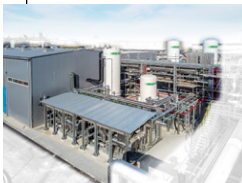
Courtesy of Depositi Italiani GNL DIG, Ravenna, Italy
