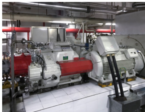
Voith VECO-Drives successfully put into operation in Guangzhou power station
