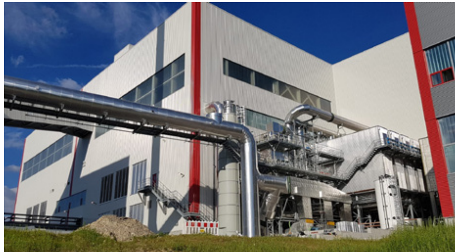
Ceramic Filter System with downstream Waste Heat Recovery, Central Germany
