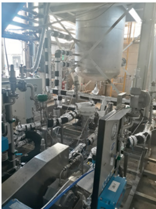
Pompe criogeniche Vanzetti Engineering VT1 per Argon liquido
