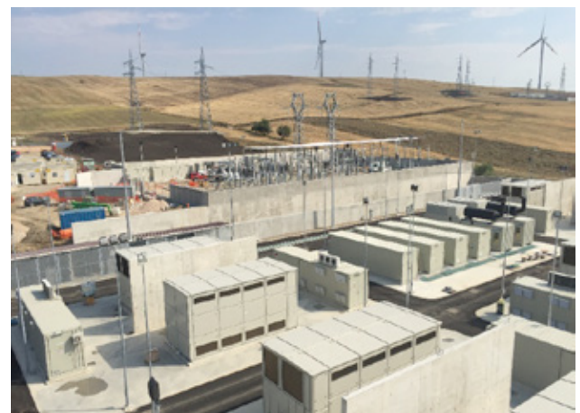
Fig. 15 SAET experience with NaS Battery (6h duration) 10.5MW-72MWh BESS in Scampitella (BN - Italy)
