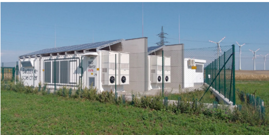
Fig 3 - Energy Storage system used for primary regulation 2.5MW-3.2MWh in Prottes (Wien - Austria)
