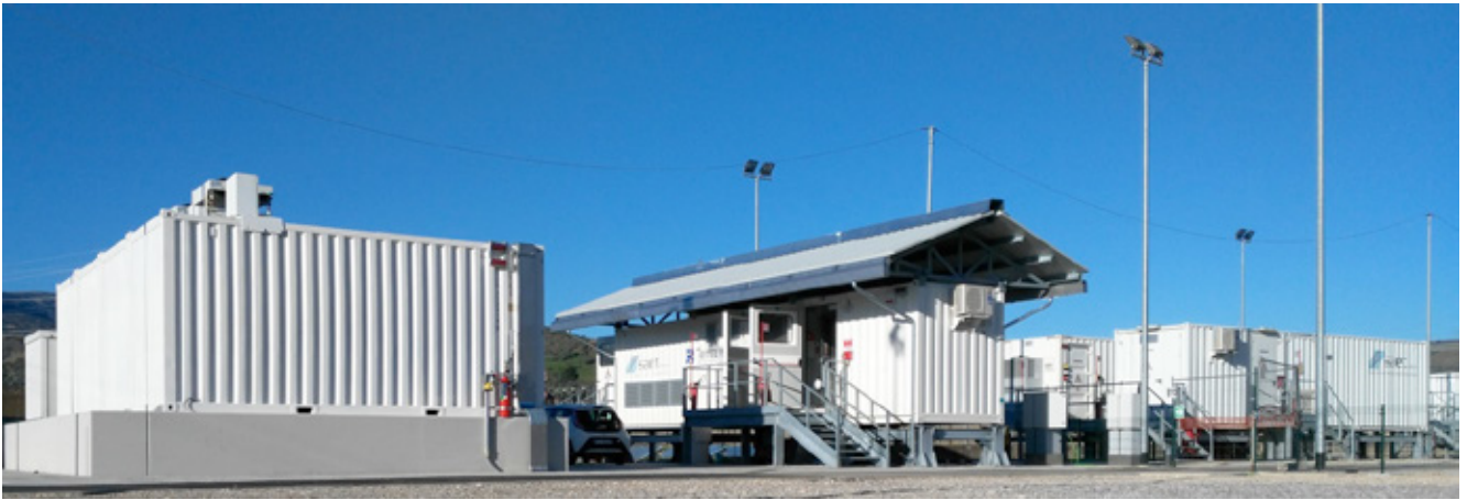
Fig. 17 - SAET experience with VANADIUM BASED energy storage system -450kW/1440kWh in Ciminna (PA-Italy)
