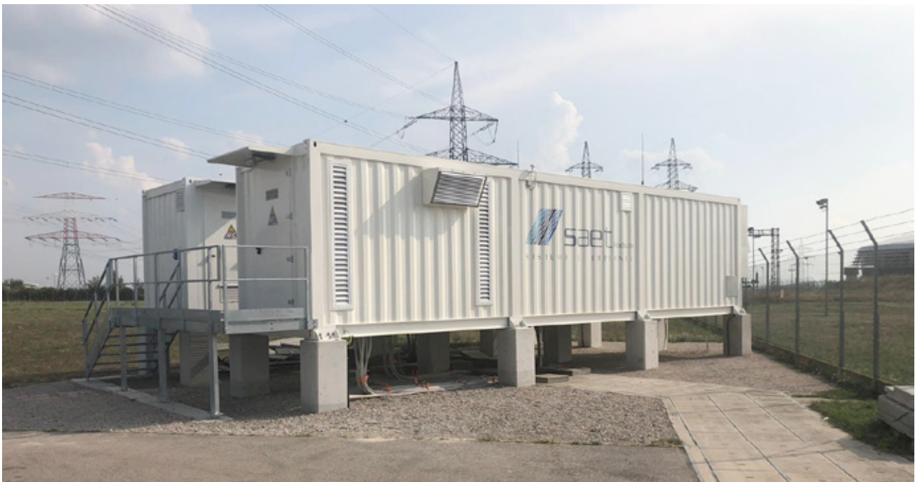
1 MW/0.5 MWh Energy Storage plant in Wien (Austria) for VERBUND Hydro Power GmbH
