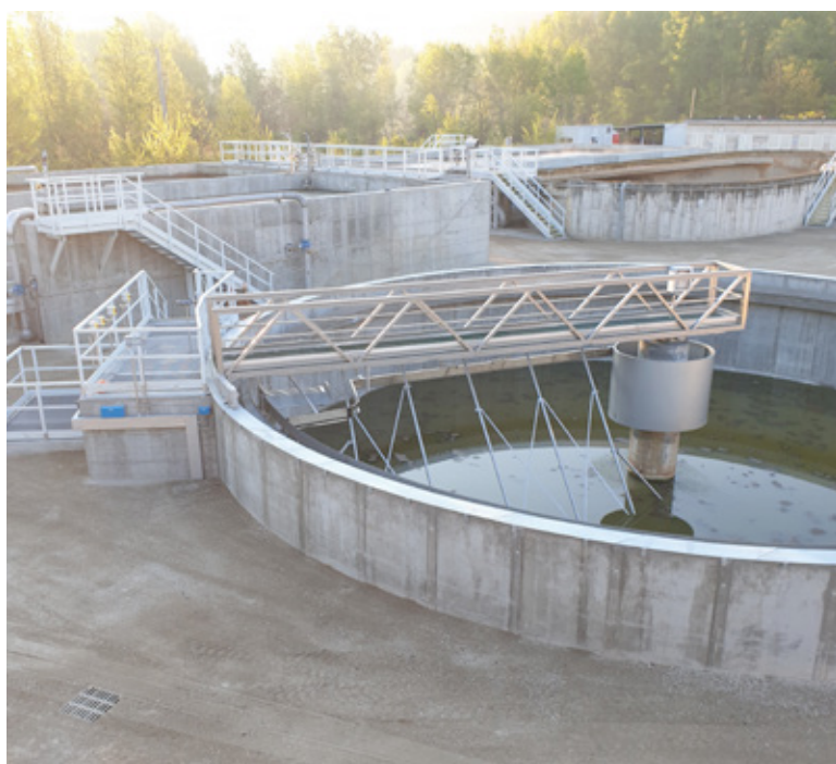
Purification plant: M.M. fibreglass structures (walkways, handrail systems and stairways)
