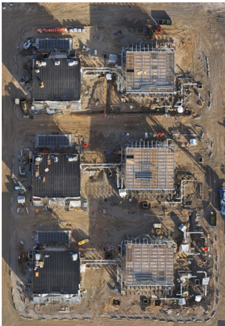
Figure 3: Aerial view of the Gas Compressor station during assembly at site. The air coolers are shown in the right side of the figure whereas the left side shows the compressors buildings. (Renco S.p.a.)
