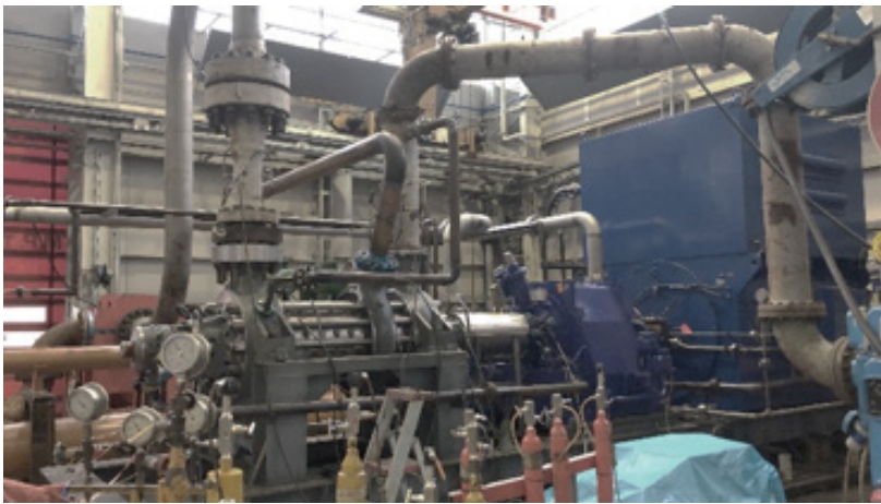
The horizontal high pressure boiler feed water pump under testing at Termomeccanica Pompe's La Spezia test center
